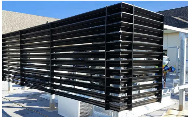
Rooftop Screening | Sharchs
