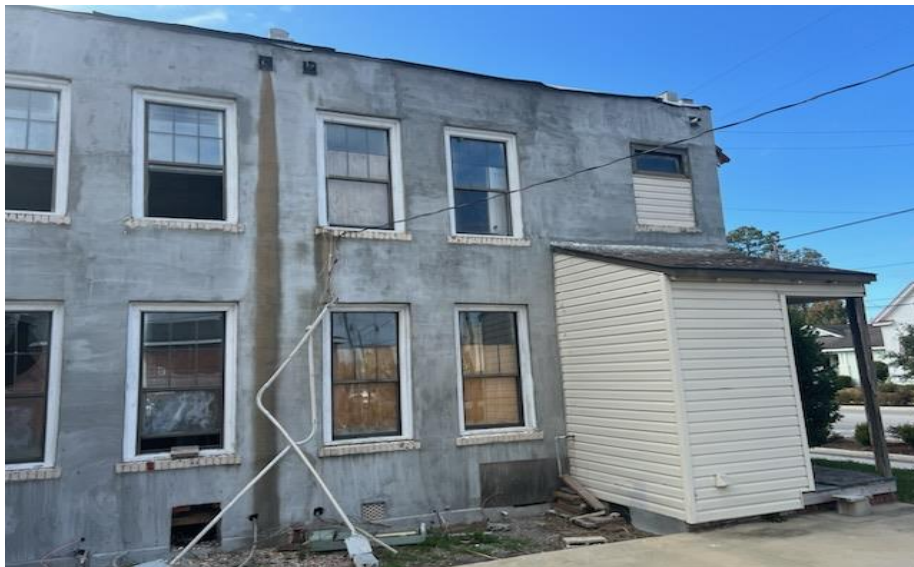
Rear façade showing attached storage building to be demolished and rebuilt for bathroom.
