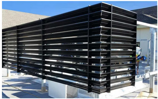
Rooftop Screening | Sharchs
