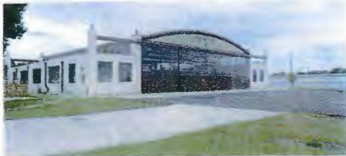
The trusses and window frames were all cleaned by hand with wire brushes and sandpaper before being restored with a rust-converting compound.
